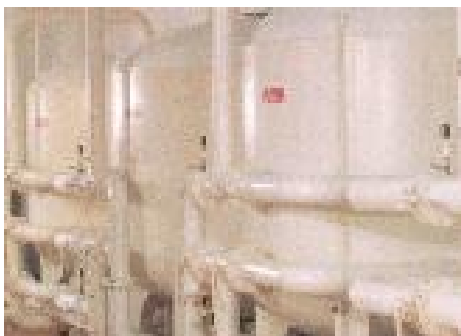
Water Treatment System
